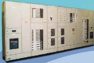
Electrical Control Panel
